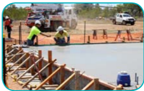
Work is well underway on the civil works at QER's Yarwun site.
